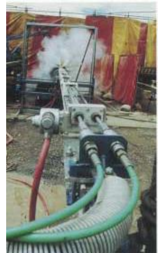
Automatic tube cleaning eliminated human contact
