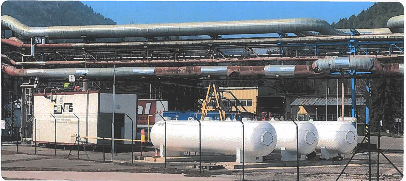
Mobile boiler room
